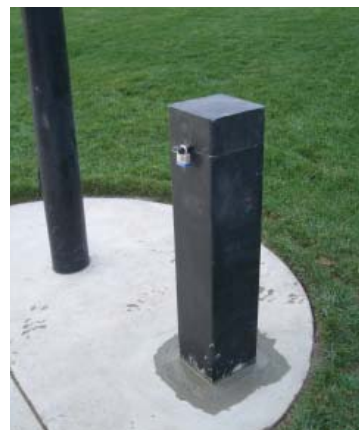
Monitoring well containment box
