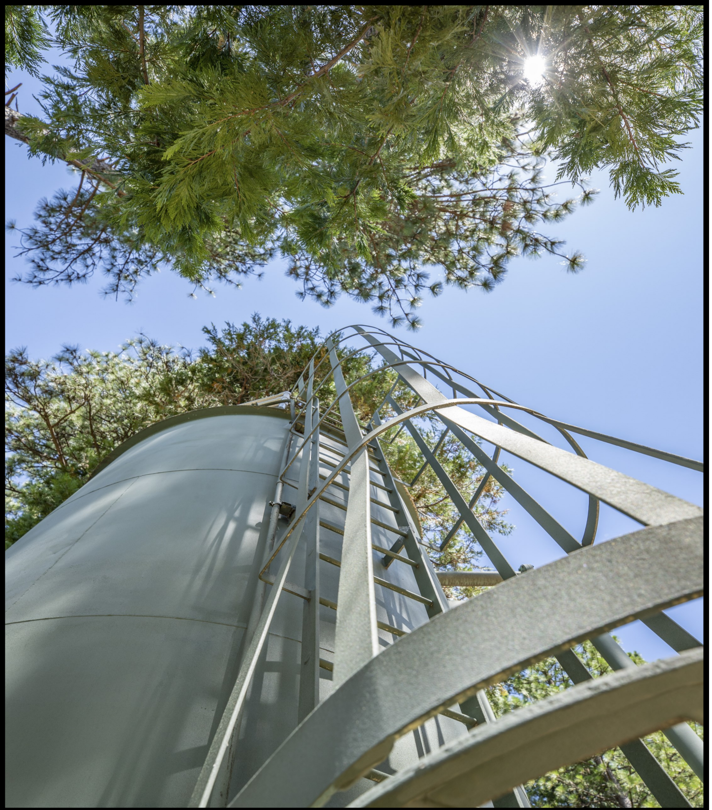
Water Tank - Alta Water Treatment Plant
